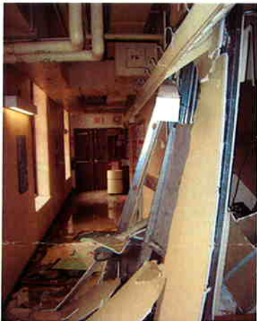
Figure 2 - Hallway Outside Laboratory Showing Explosion Damage
